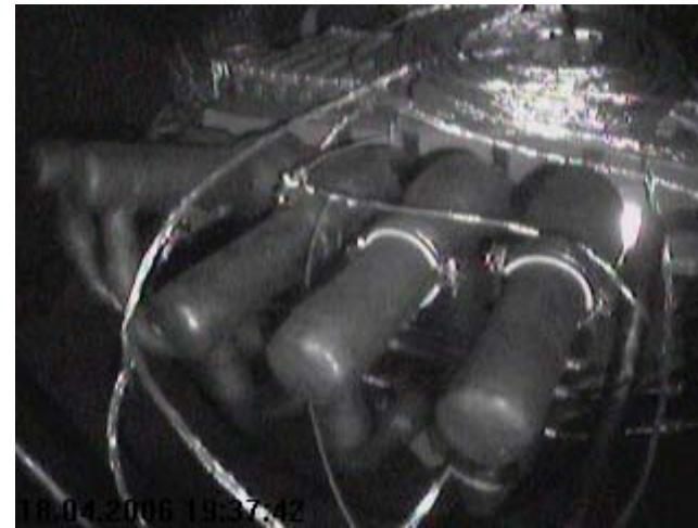
2. Discharges in the region of the insulation defect visible with video system
