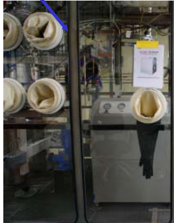
2x Electrolyser each 1 m 3 /h
